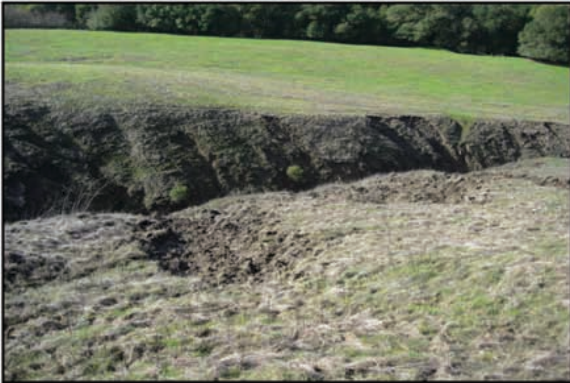
Photo 9: Eroded Slope Following Heavy Rains, Tributary to Rodeo Creek (June 2006)
