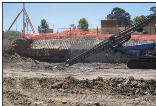
Some of the dirt was transferred to the future site of Duck Pond Park for reuse
