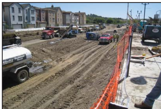
Crews worked for five months to remove dirt and install soil nail walls to prepare for construction of the underground parking
