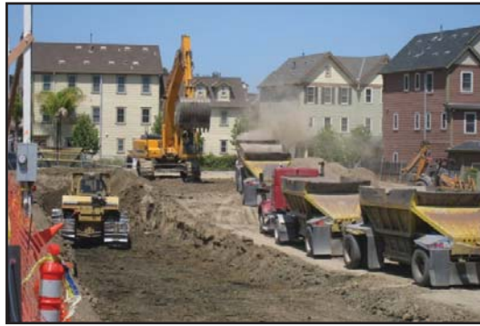
Close to 50,000 tons of dirt was removed to make way for underground parking
