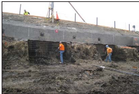
Shoring walls protect the site from groundwater until permanent retaining walls are constructed
